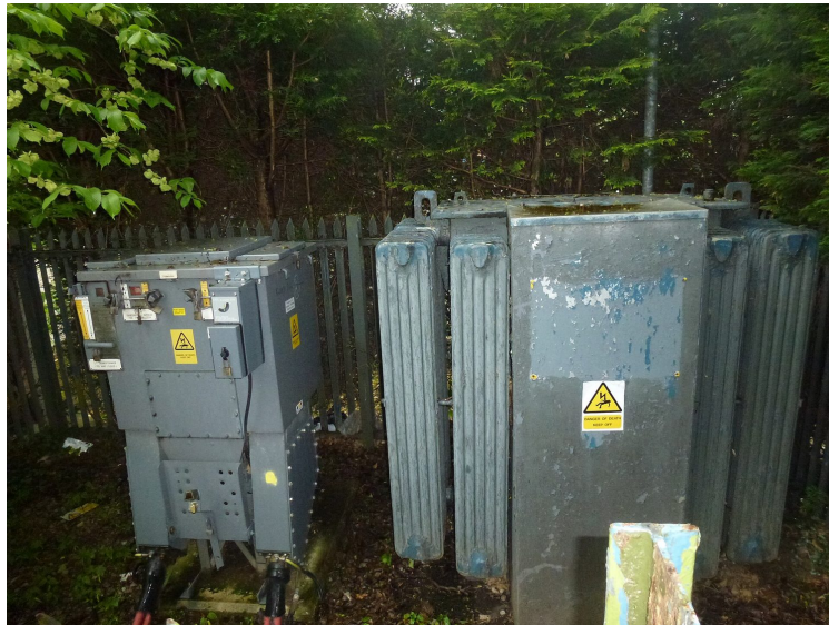
A substation's transformers step alternating voltage up or down.
